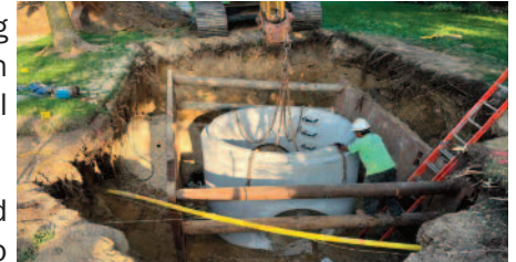
Road improvements in the Willoughby Farms Subdivision will be financed through the Village's 2024 bond issuance
