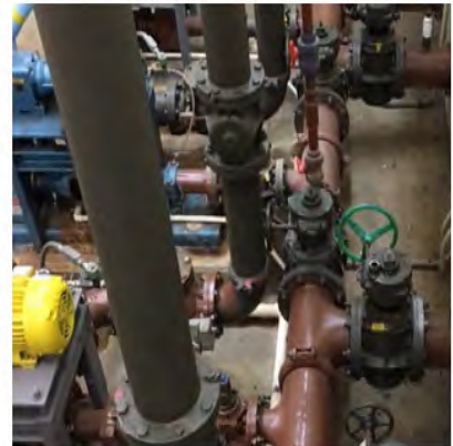
Primary Sludge Pumping Improvements brings automation to solids handling at the WWTF.
